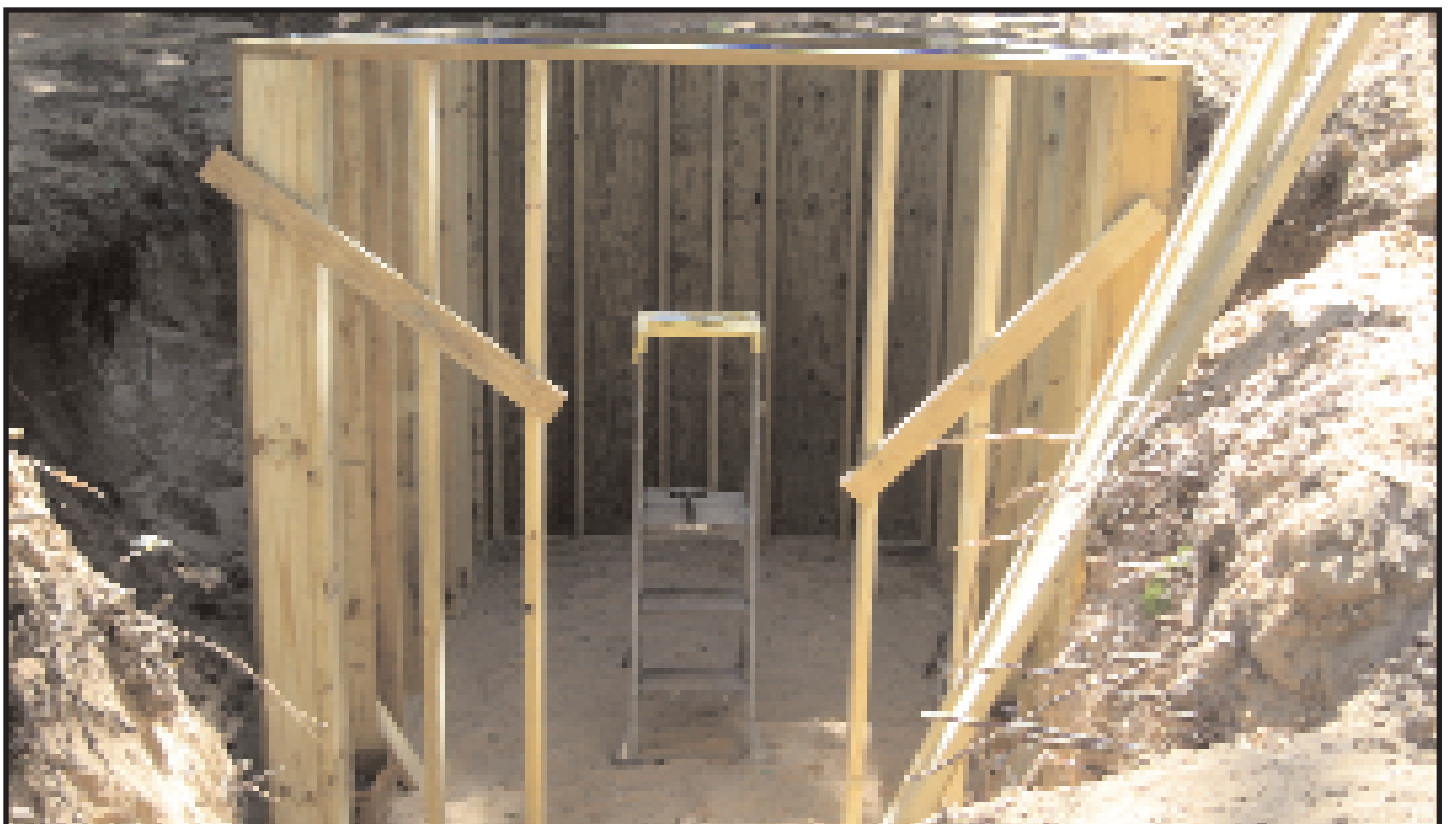
Root Cellar under Construction. The ladder in the center gives an idea of the size of the underground storage area for our home grown produce. Come and see the finished product at the July 14 Member Meeting.
